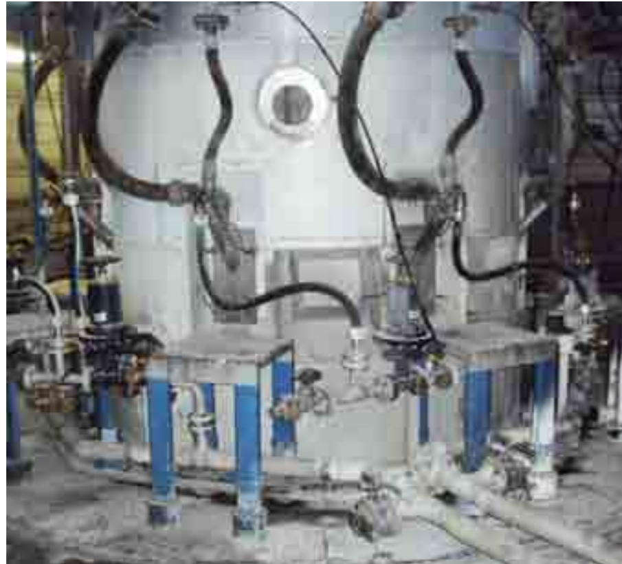
Twin-fluid nozzle lances in an existing system, with tables for the frequently necessary disassembly and cleaning of the nozzle lances
